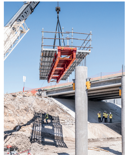
Access safety is built-in before lifting and installation of the cap system.
